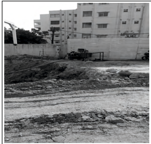
Fig. 4. (b) Barricade is not provided on construction site
