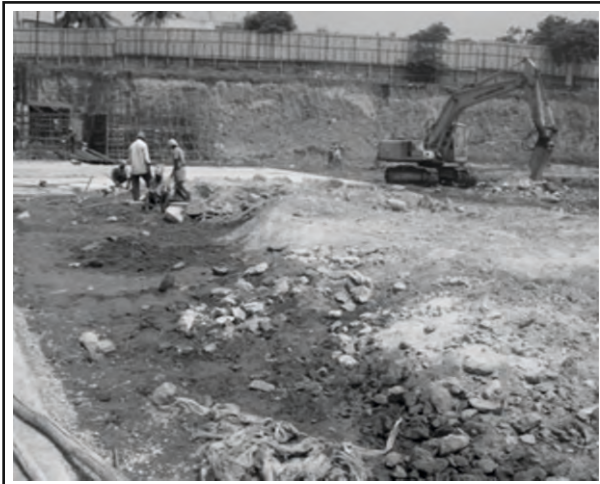
(e) Improper stacking of soil
