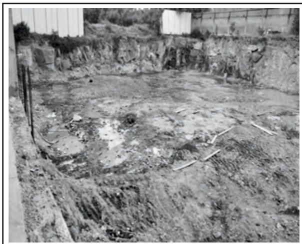
(h) Seepage of water
