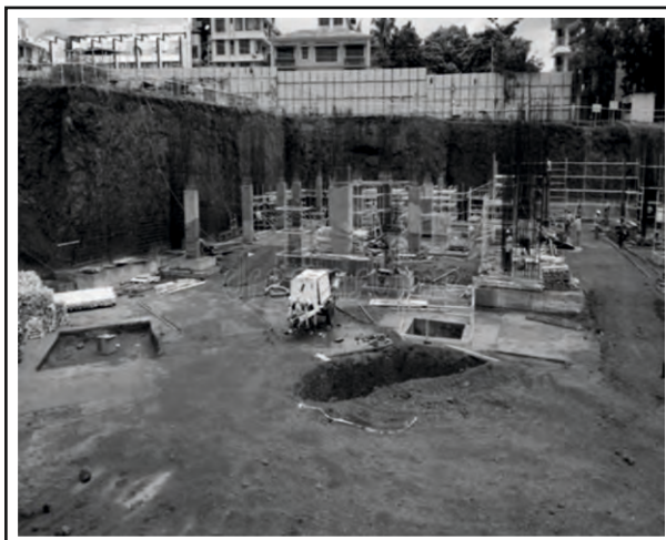
(g) Improper barrication
